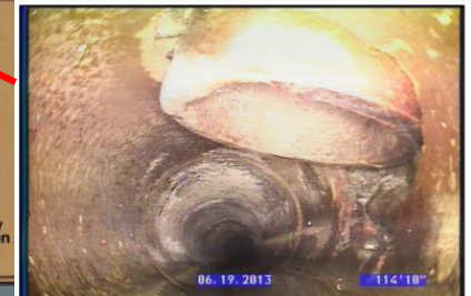
Photo: 20_20_172_A.JPG, Media No.: 120613_1, 00:04:37 114.65FT, Tap Break-Intruding, at 02 o'clock, 4", 2", within 8 inches of joint: YES
